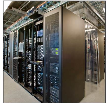
Server towers with racks
