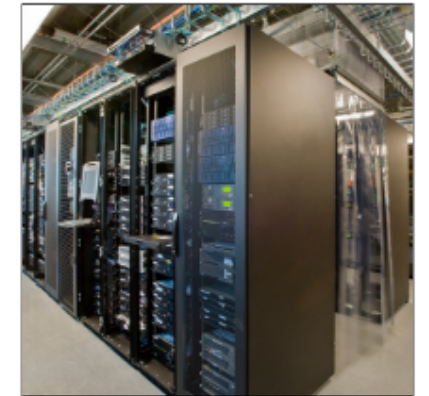
Server towers with racks
